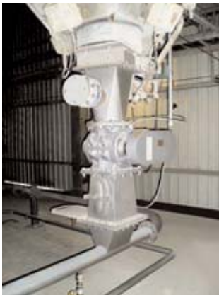
FLUIDCON transport system at E-on Farge Plant
