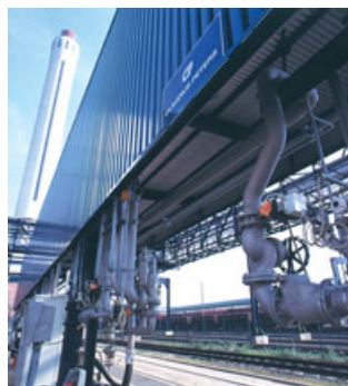
Limestone unloading station
