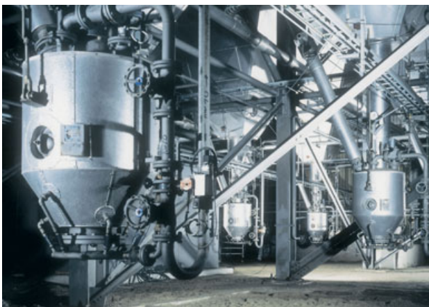
Pressure vessel ash collecting system
