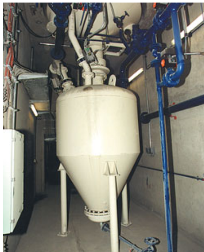
Ash transport pressure vessel
