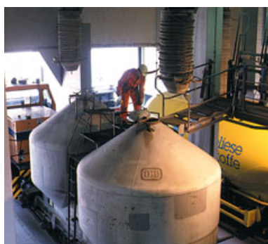
Tank wagon loading of fly ash
