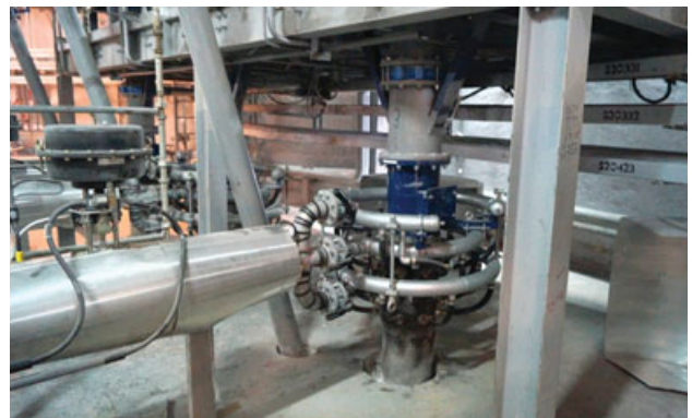
Humidification station for 340 t/h fly ash
