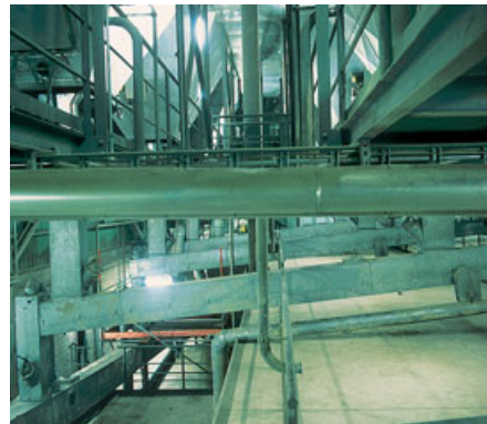
Ash collecting aeroslide system beneath the ESP
