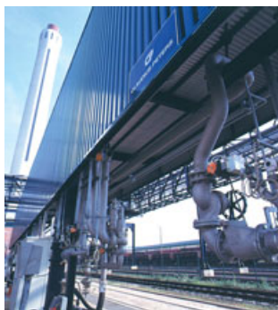
Limestone unloading station
