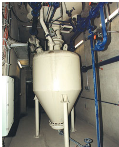
Ash transport pressure vessel
