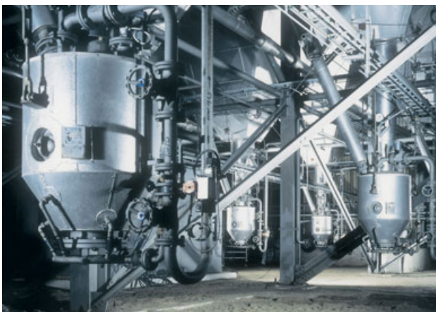
Pressure vessel ash collecting system
