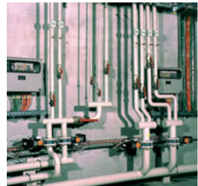
New installation of air distribution system for silo aeration including electro pneumatic flaps
