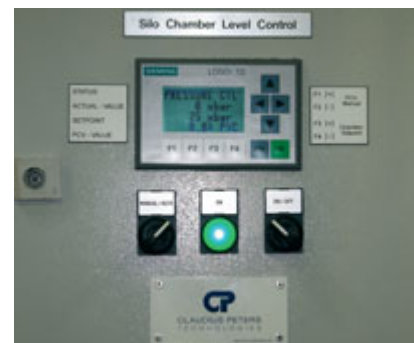
③ Local control panel
