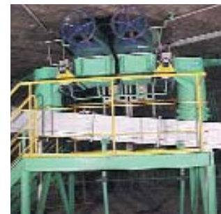
Flow control gates
