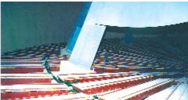
Steel mixing expansion chamber, retrofitted in old silo
