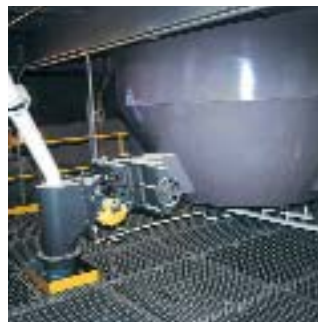
Collecting bin, discharge
