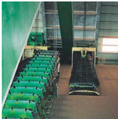
Reclaiming: scraping arm
