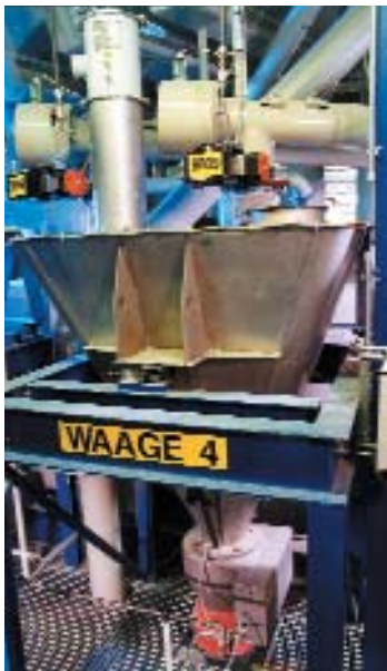
Mixing system for batch operation
