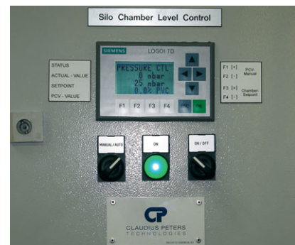
③ Local control panel
