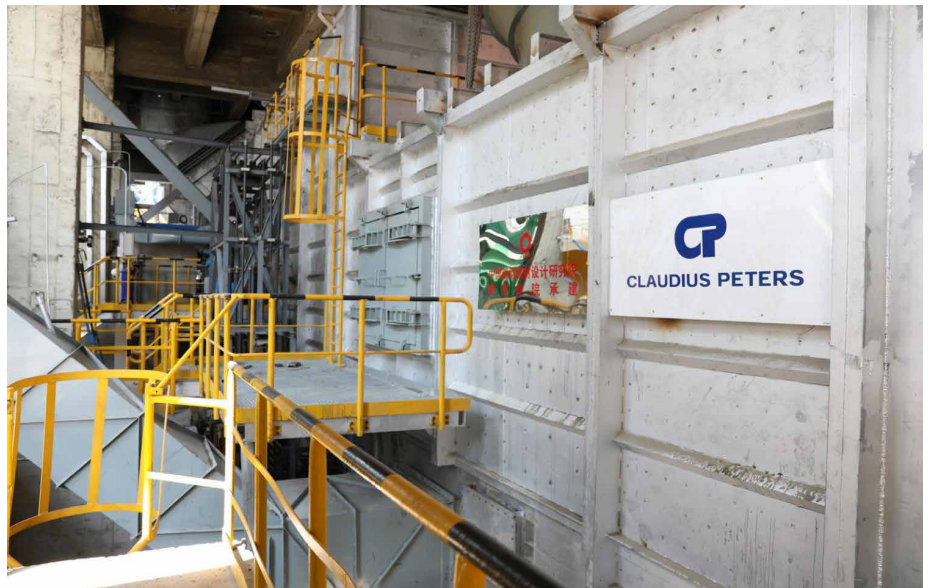
ETA Cooler. Plant: Shanshui Pingyin Line #2, Clinker Capacity: 6500 t/d, in operation since April 2020.
